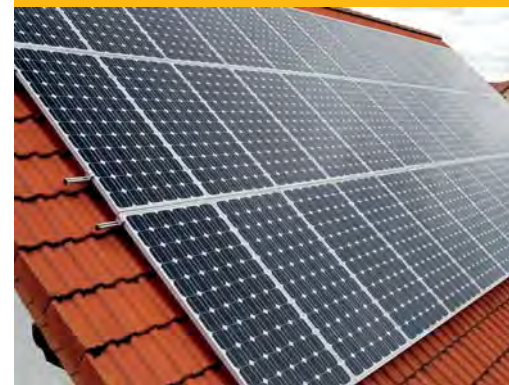
Roof-mounted solar modules
